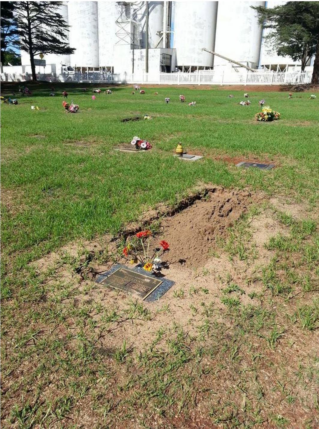
A sinking grave at the Toowoomba and Drayton Cemetery.
